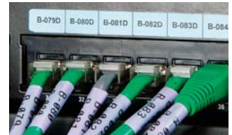
Patch Panel Labels
